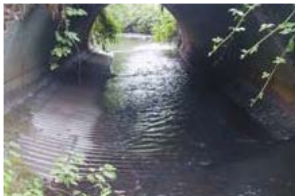
Low flow through Ames Creek culvert
