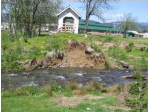
Bank erosion on Ames Creek
